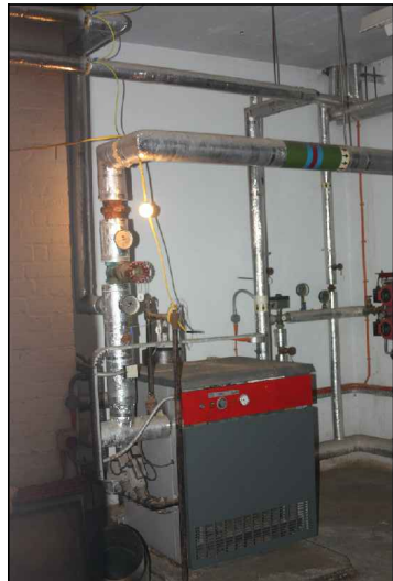
DP 1: Basement Boiler Room - View NW
